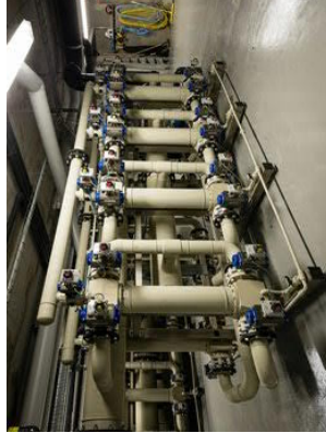
Figure 17 - Ceramic Silicon Carbide Pool Filtration system (courtesy of LiqTech)
